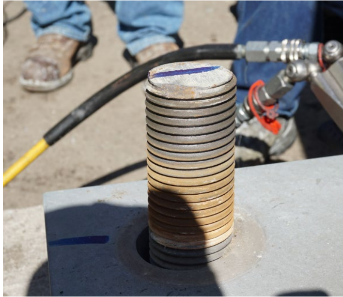
Figure 3.2.12. Rod 10 out of plumb and misaligned
