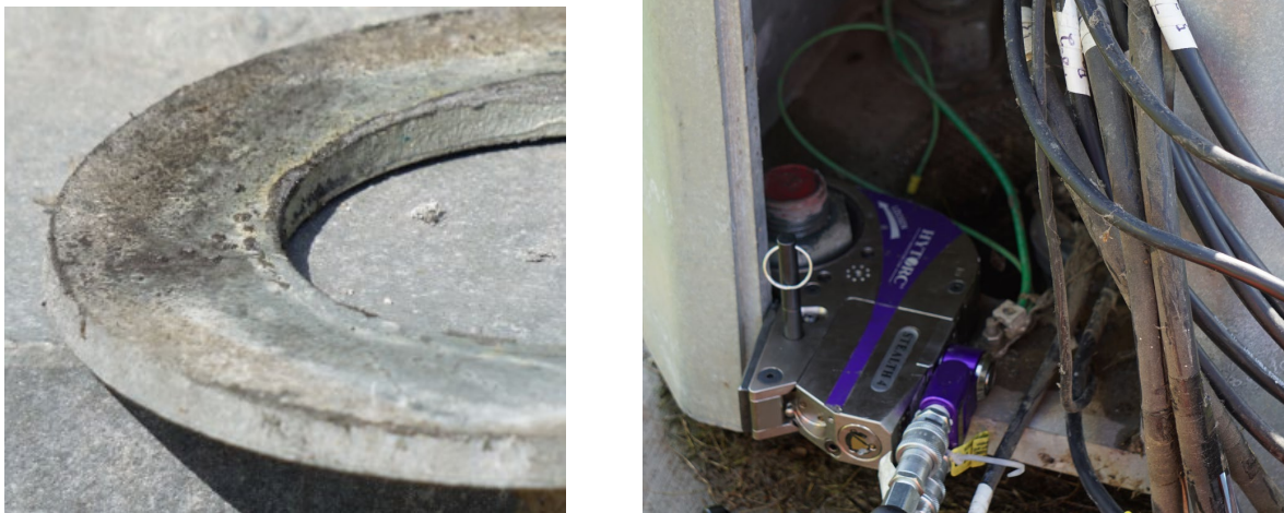
Figure 3.3.13. Galvanizing dimples on washer (left) and moved grounding wire (right)
