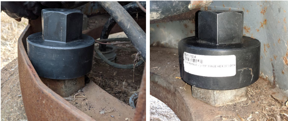
Figure 3.3.18. Wedging on door frame (left) and socket raised into wall by nut protrusion (right)
