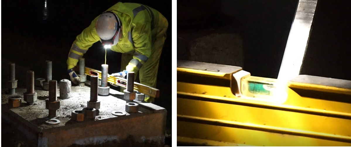
Figure 3.2.2. Leveling nuts on sign truss structure (left) and final installation of COSS out of plumb (right)
