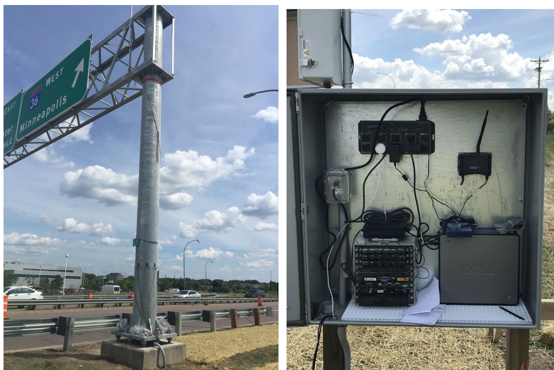
Figure 4.1.1 Instrumented sign post (left) and data logger cabinet (right)
