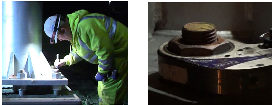
Figure 3.2.5. Marking each rod and nut as reference for the turn-of-nut tightening (left) and tightening using a hydraulic wrench (right)
