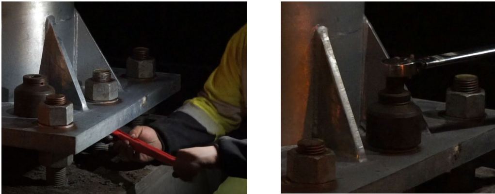
Figure 3.2.4. Tightening leveling nuts with pipe wrench (left) and snugging top nuts with a calibrated wrench (right)
