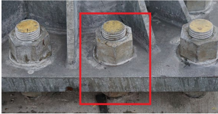
Figure 3.2.6. Out-of-plumb anchor rod on COSS OH 280-023
