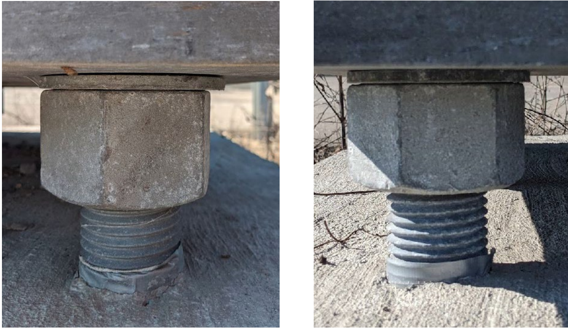
Figure 3.2.7. Gap between baseplate and washer #5 out of plumb (left) and bolt #8 plumb for reference (right)
