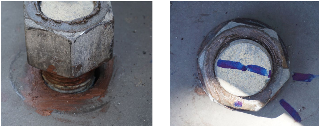
Figure 3.2.15. Missing washer on rod 8 (left) and excessive turn of nut on rod 11 (right)
